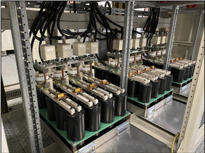
Figure 3 - Snubber installed at the bottom of CT2 ATLAS Toroid breaker box.
